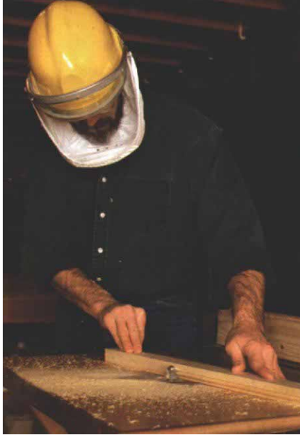
You can keep the beard. As this bearded trim carpenter runs moldings on a router table, filtered air from a belt-mounted battery pack washes across the inside of his face shield. The Tyvek face guard helps keep dust particles from entering below the shield.
